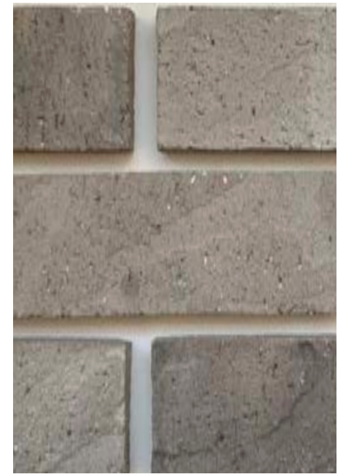
WEATHERED BRICK 2 SAMPLE
